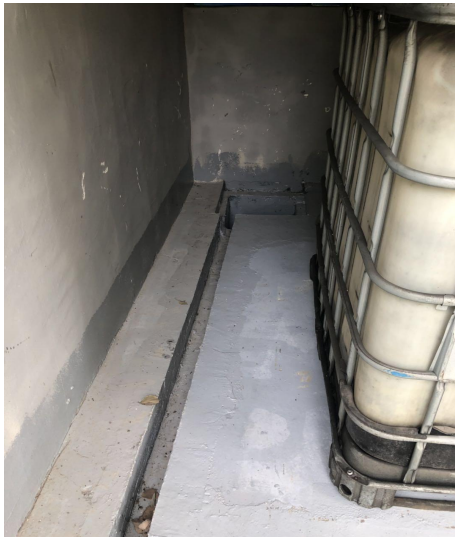
危废仓库导流沟、集液池、环氧地坪
